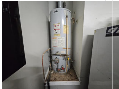
Water Heater Garage
