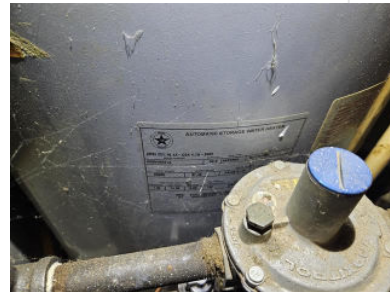
Water Heater Data Plate
