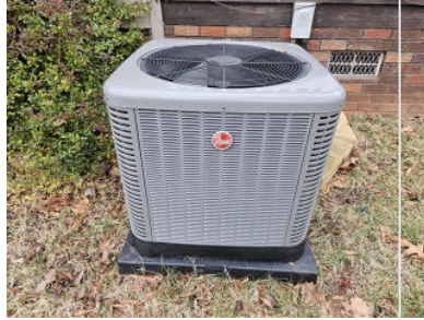
Air Condensing Unit
