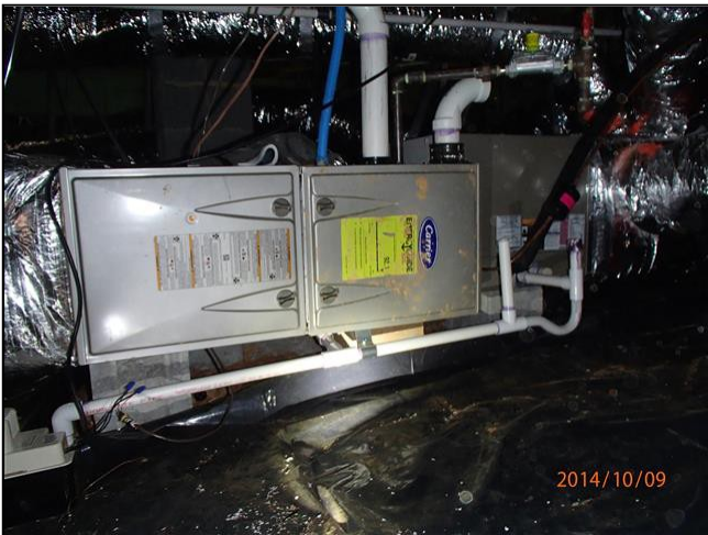
Gas Furnace (Crawl Space)
