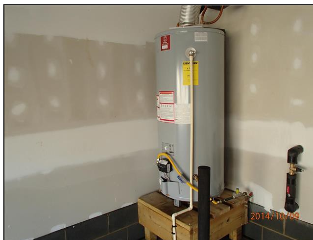
Gas Water Heater
