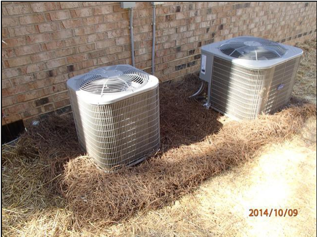
AC condensing unit (Outside)
