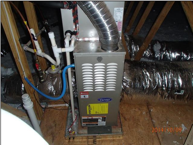
Gas Furnace (attic)
