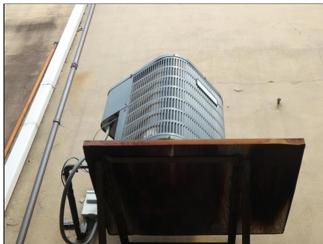
AC Condensing Unit (Outside Unit)
