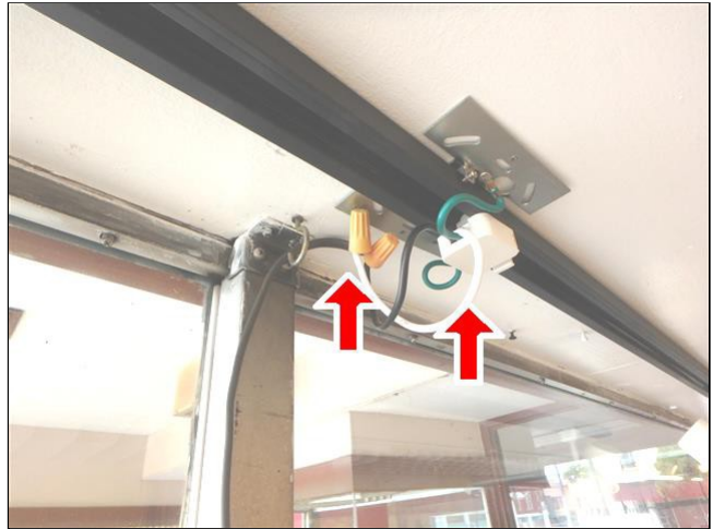
6.4 Item 2(Picture) Exposed Branch Wiring.
