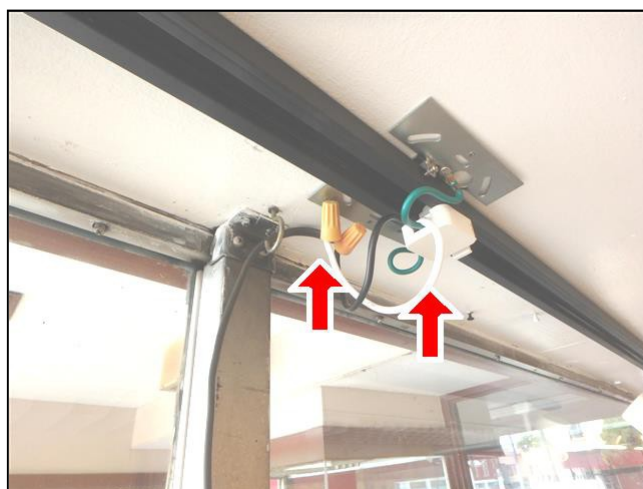
6.4 Item 2(Picture) Exposed Branch Wiring.
