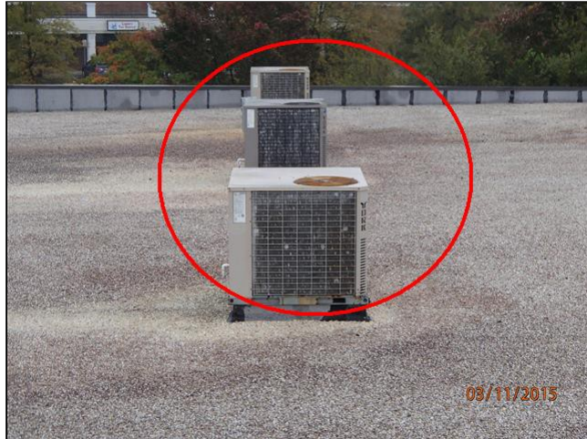
8.0 Item 1(Picture) Heat Pump
