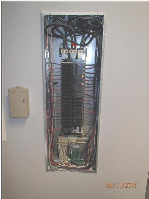
6.0 Item 1(Picture) Electrical Panel With Cover Off (Unit 3710B)
