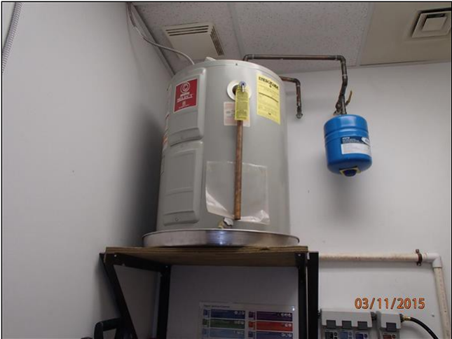
Electric Water Heater (Unit 3710)
