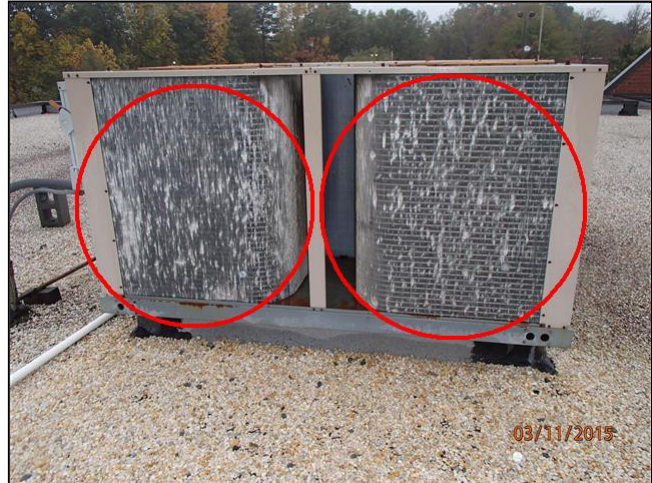
8.0 Item 2(Picture) Package Units
