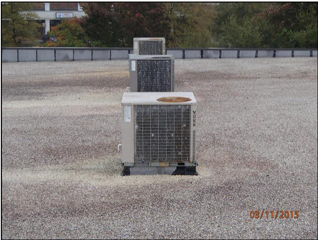
Heat Pumps (Unit 3710-B) NOT INSPECTED
