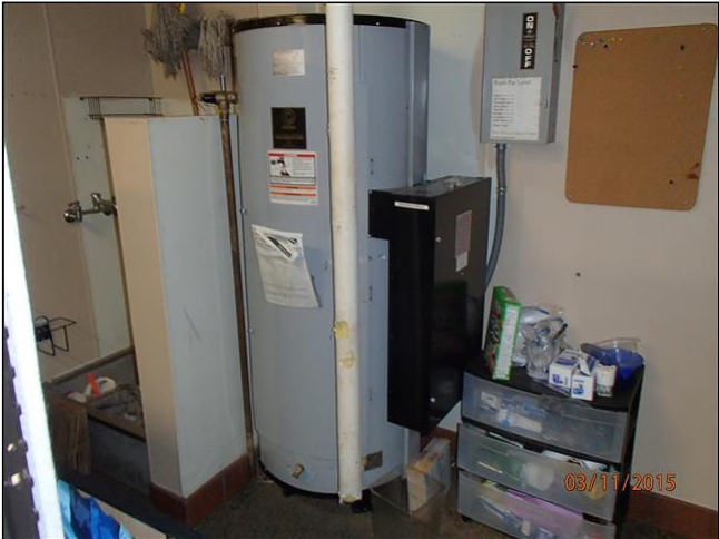
Water Heater (Unit 3710-A)
