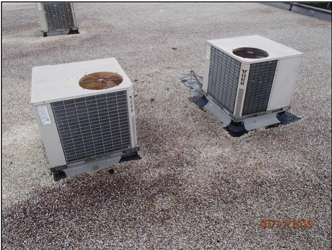
Heat Pumps (Unit 3710-A)
