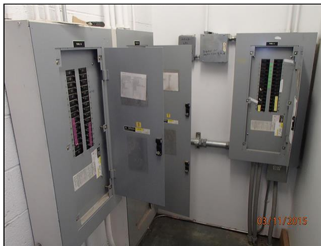
6.0 Item 3(Picture) Electrical Panels (Unit 3710 Goodwill)
