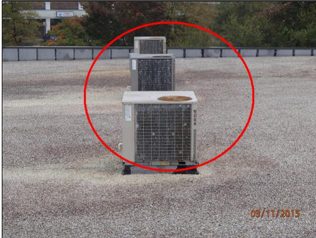
8.0 Item 1(Picture) Heat Pump
