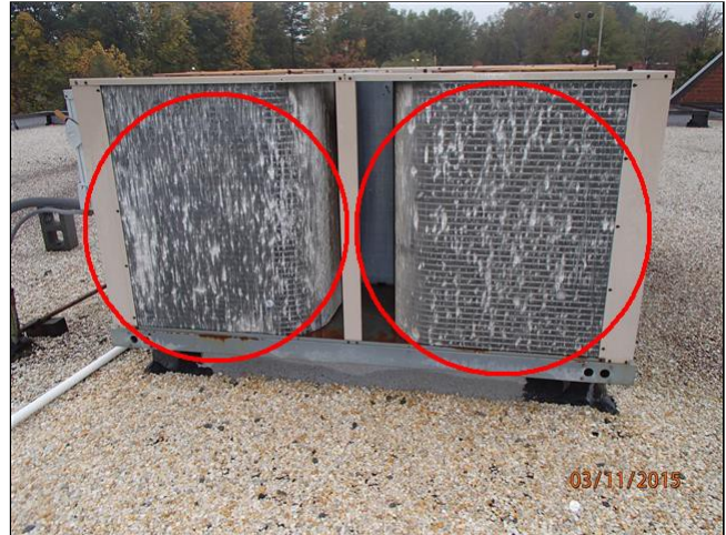
8.0 Item 2(Picture) Package Units
