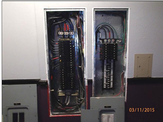
6.0 Item 2(Picture) Electrical Panels (Covers Off) Unit 3710-A
