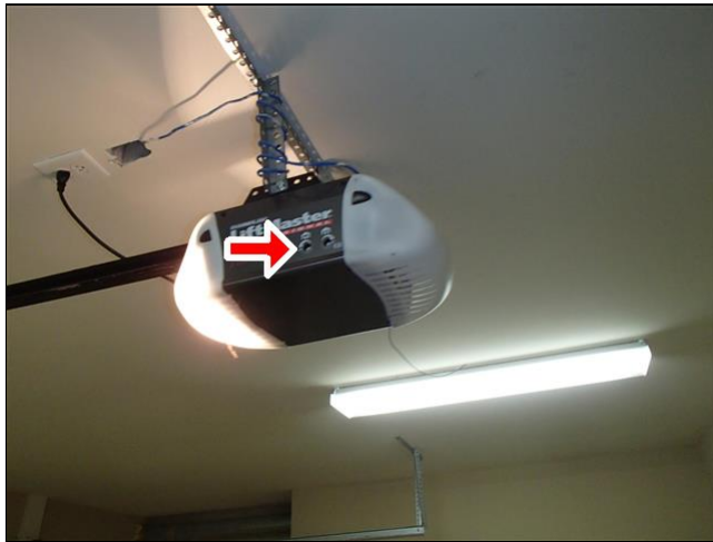
Basement Garage Door Operator
