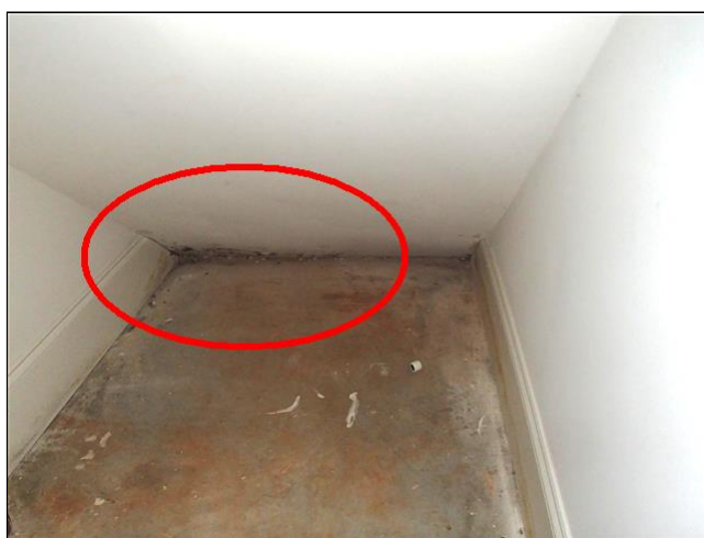
From Shower Pan Leak
