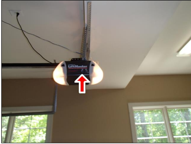
Left Garage Door Operator
