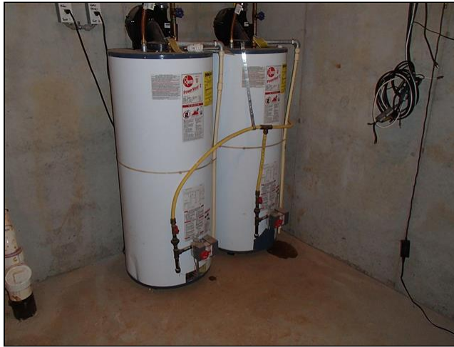
Gas Water Heaters (Basement)
