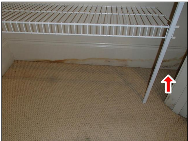
From Shower Pan Leak
