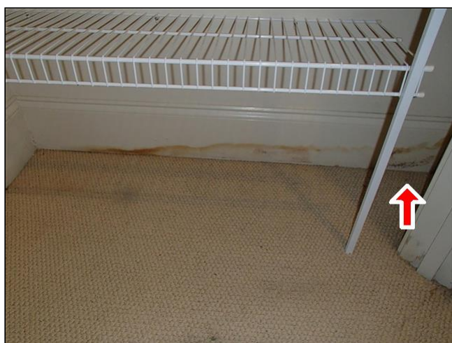
From Shower Pan Leak
