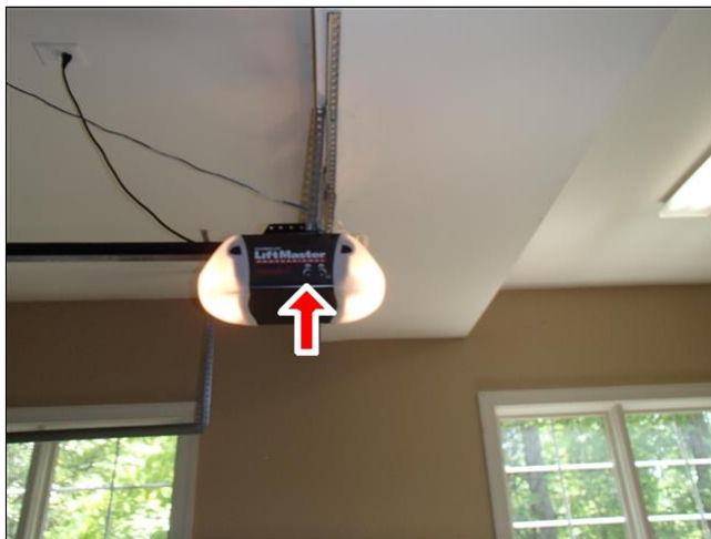
Left Garage Door Operator
