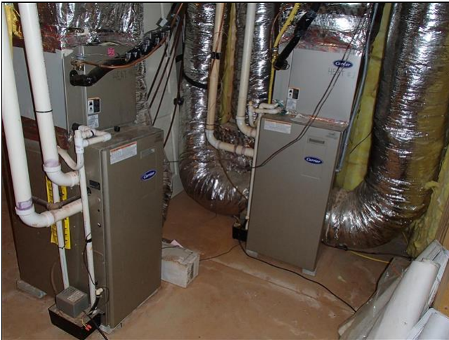
Gas Furnace(s) Basement 1st floor & Basement units
