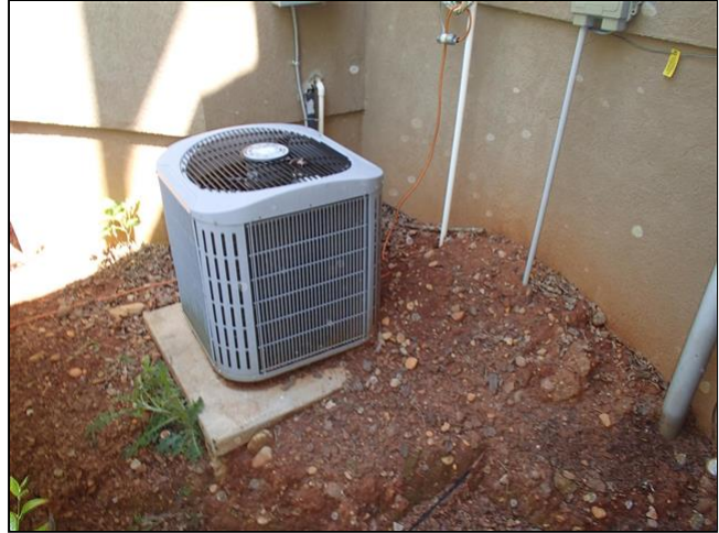
AC condensing Unit (Outside) 2nd floor unit
