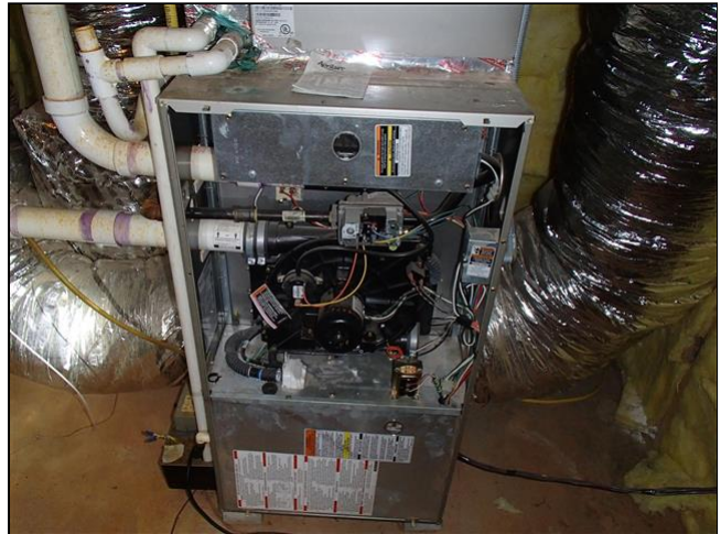
Gas Furnace (Cover Off) 1st floor unit
