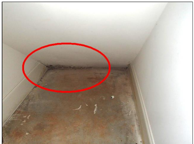
From Shower Pan Leak
