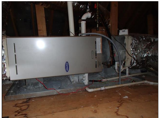
Gas Furnace (Attic) 2nd floor unit
