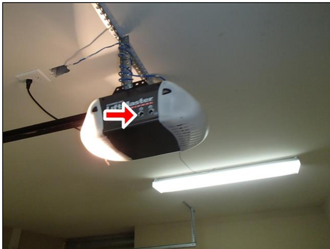
Basement Garage Door Operator
