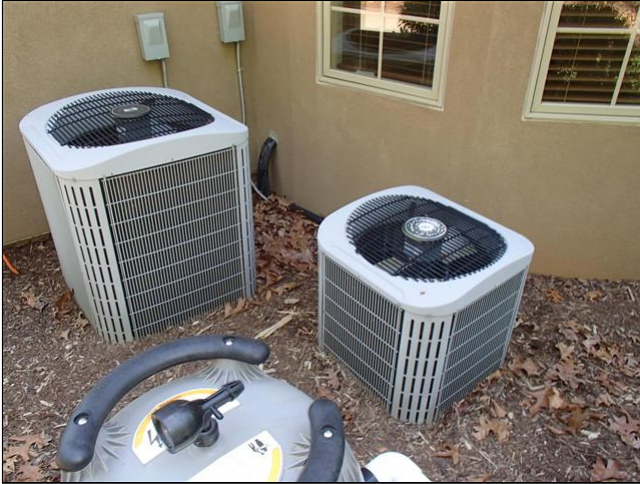
AC condensing Units (Outside) Basement and First Floor Unit
