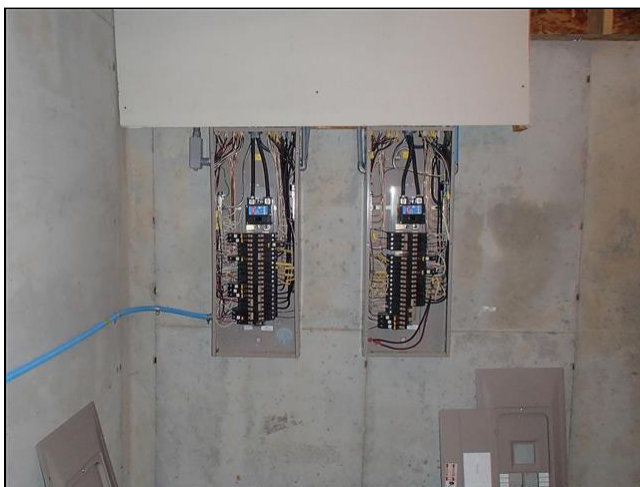
Electrical Panels with covers off
